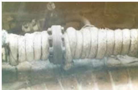
Asbestos rope used as insulation on a pipe
