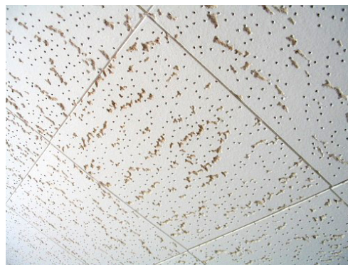
Asbestos containing ceiling tiles
