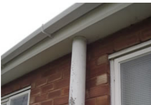
Asbestos cement drainage pipe (downpipe)
