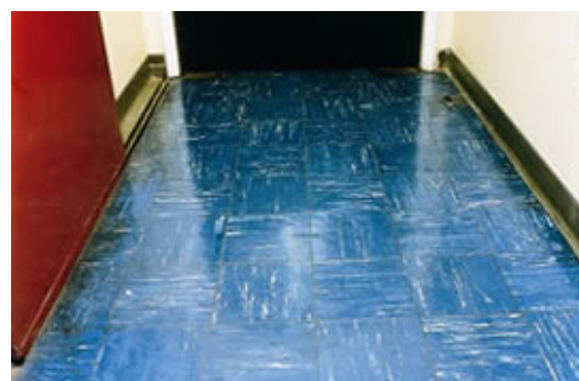
Asbestos containing floor tiles in a corridor
