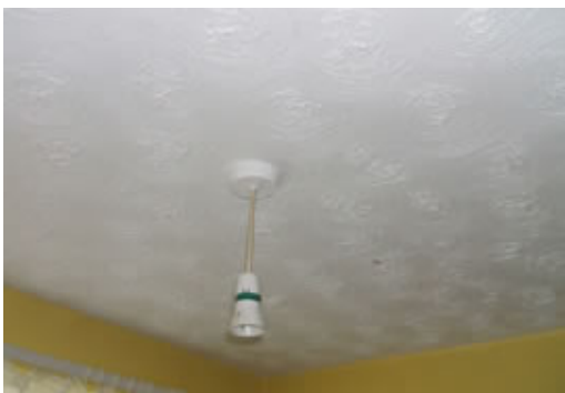
Asbestos textured coating
