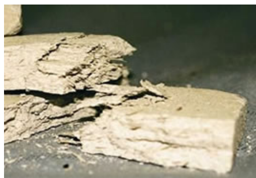
Pieces of Asbestos Insulating Board (AIB)
